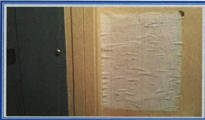
# 3 HUD placard located in master closet; right of the main electrical panel.
